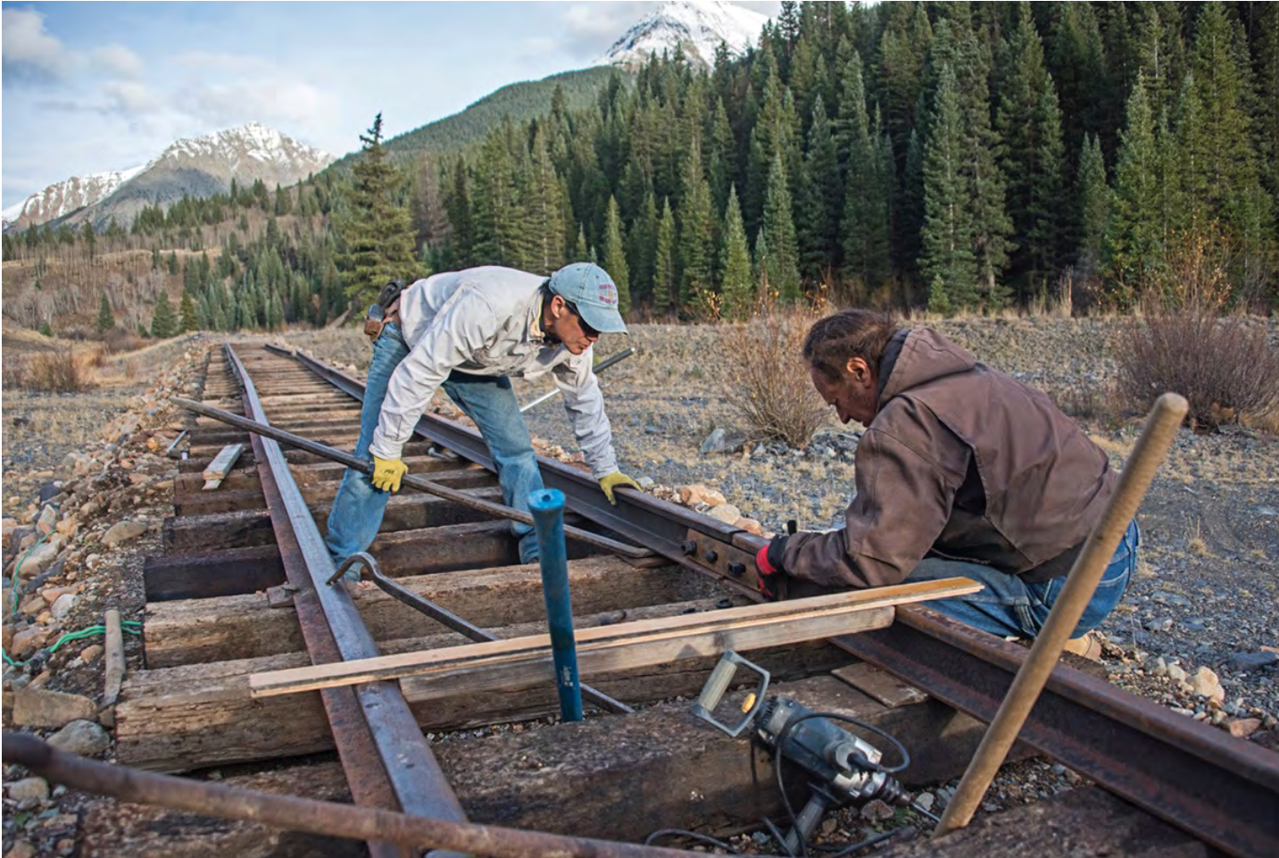
Beneath the snow covered peaks of Galena Mountain and Little Giant Peak, Loren Lew (left) and Mike Geryak align rail on the first segment of the planned Silverton Northern rail project in a work outing last fall. A full 220 feet of rail was laid on the way to the first goal of Arastra Gulch. It is perhaps the most ambitious project ever undertaken by the Society which is known for biting off big chunks and actually getting them chewed!
