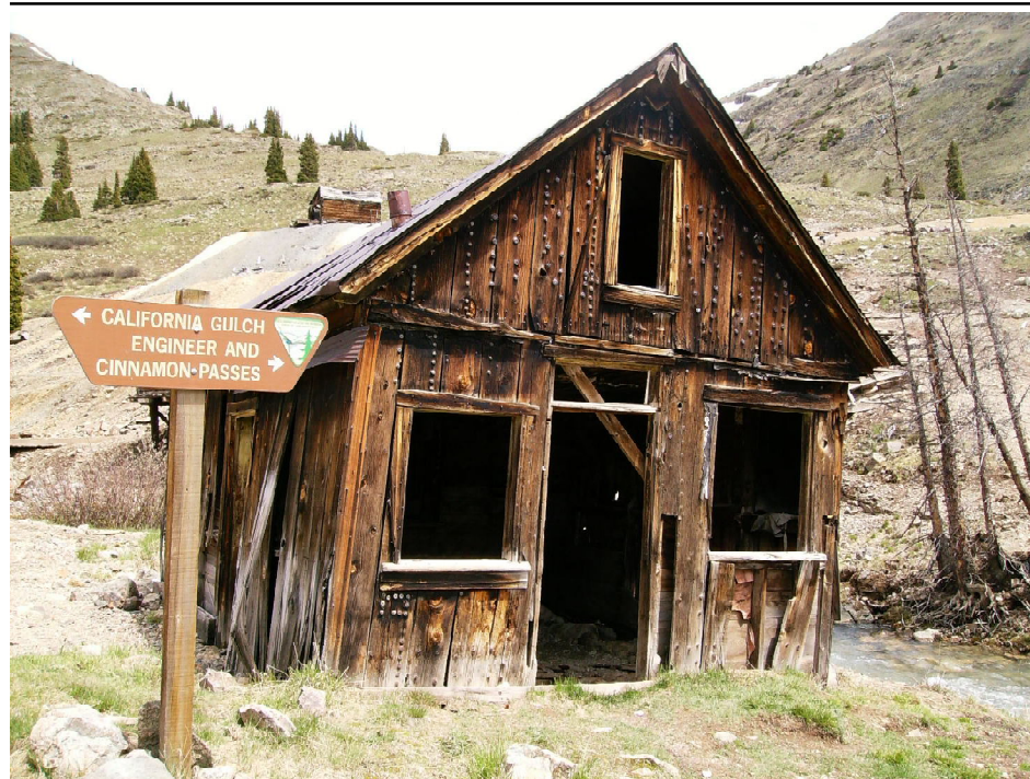
This post-1890 building in Animas Forks is at the confluence of the east and west forks of the Animas River and is one of the buildings involved in the upcoming project.
