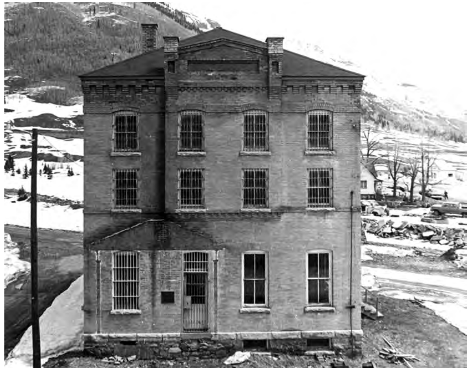
Fifteen years after opening as a museum, the 1902 jail suffered a major setback when the heavy snows of the 1978-79 winter collapsed the roof of the building, forcing temporary museum relocation itoa house on Greene Street while repairs were made. This 1981 picture shows the new roof on what appears to be a neglected building. The facing porch on the southwest side had been destroyed in an unfortunate collision with a motor vehicle.
